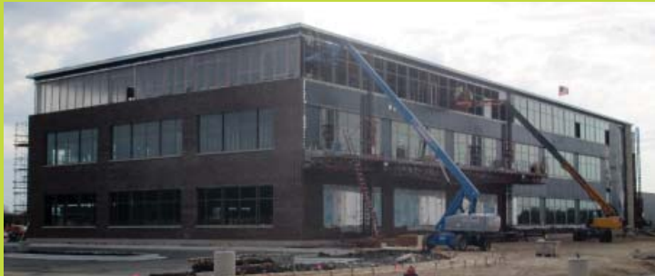
The new Aurora Cancer Care center is part of a larger Aurora Health Center being built near Spring Valley Road and Highway 36.
